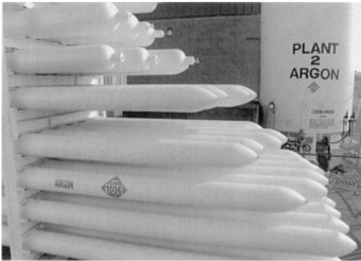
Fig. 5 Liquid argon storage and tube bank storage for argon gas. Courtesy of Bodycote IMT, Inc.
